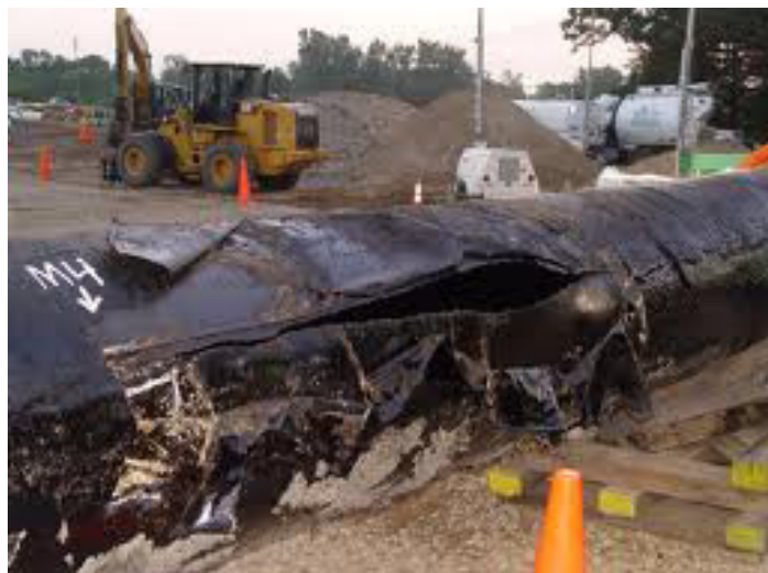
Cleaning up the 2010 pipeline spill in Marshal, Michigan (Kalamazoo) has cost almost $1 billion and is still not finished.
